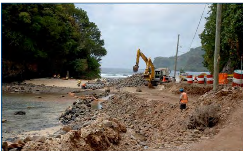
Photo 19: Road construction is an example of coastal development that can lead to anthropogenic stress on the territory's coral reef and shoreline resources. Photo: Irene Kelly, NOAA Fisheries.
